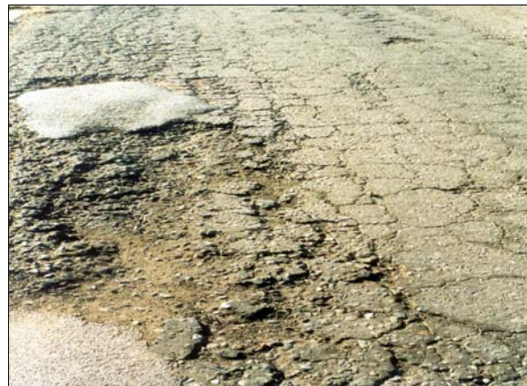
Photo 1.1. Deteriorated roadway asphalt pavement in Fort Barry.
