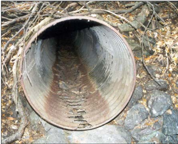
Photo 1.2. Rusted culvert under East Road.
