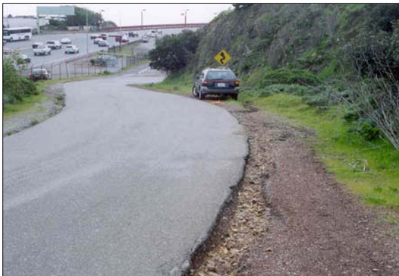
Photo 1.6. Typical unpaved shoulder parking and resultant soil erosion.
